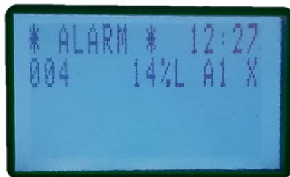
Figure 22) Screen in Alarm status
