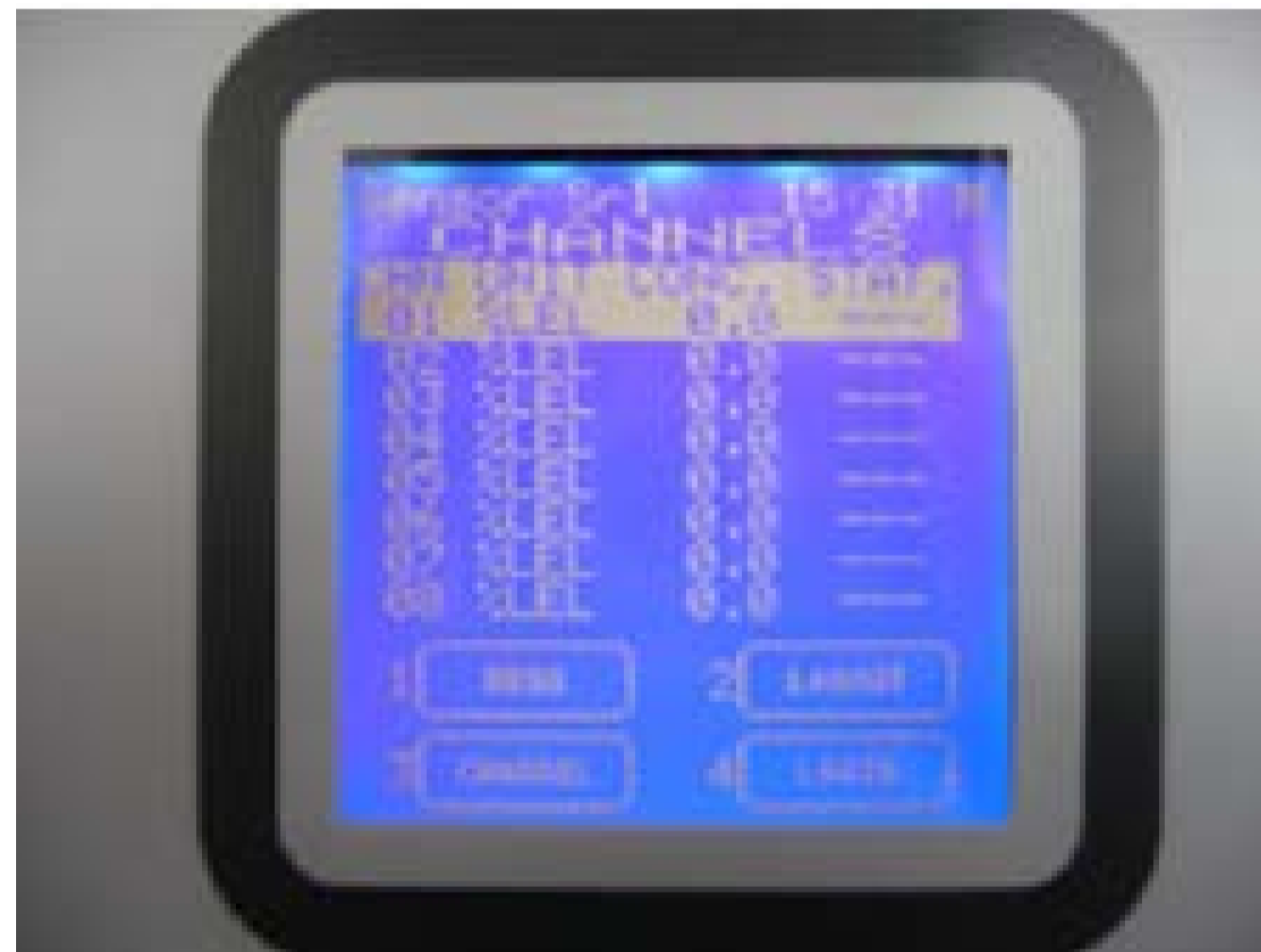
Figure 5.1.4 b) View channels screen in "Maintenance" or "Engineer" level
