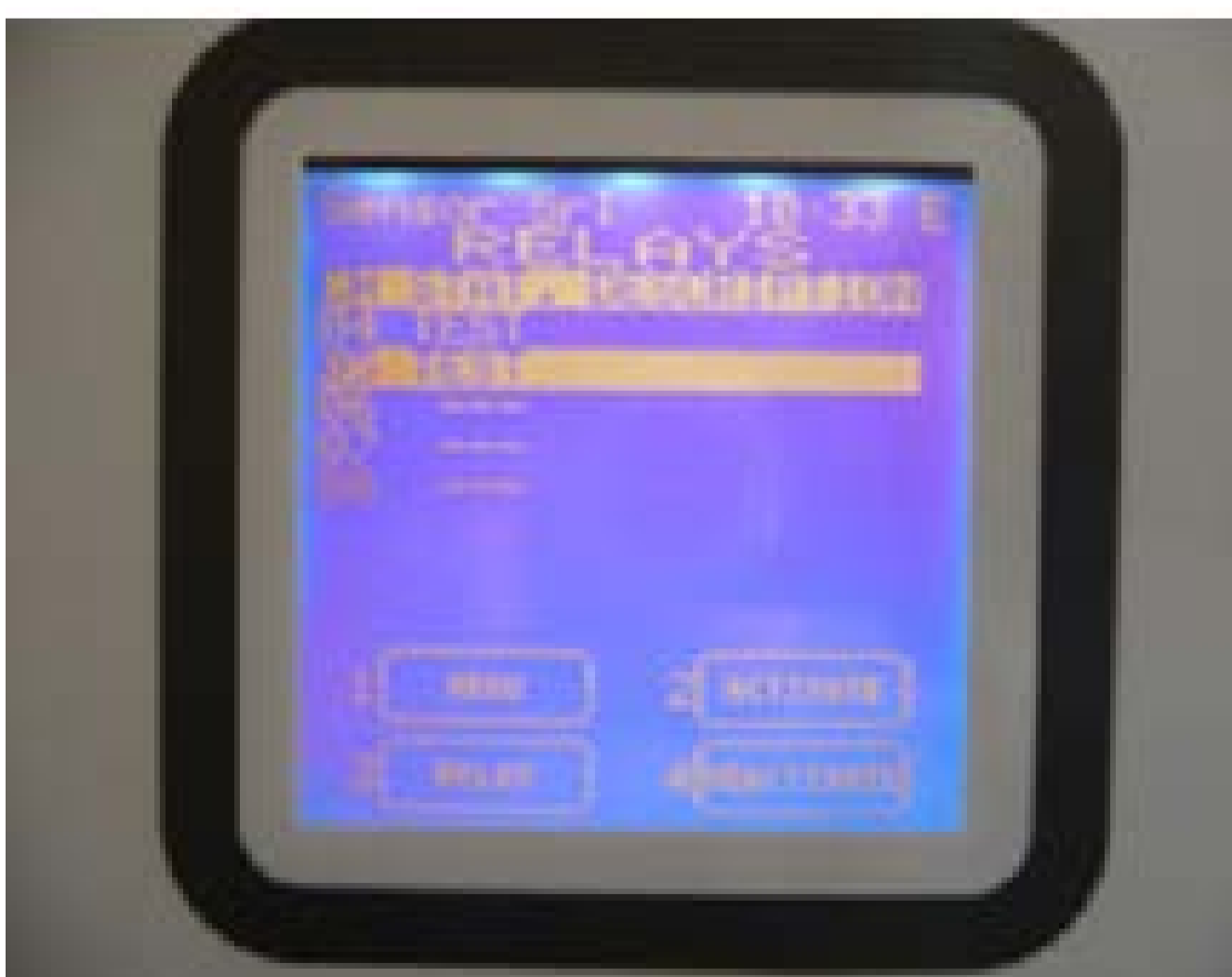
Figure 5.1.3 d) Screen with relays in “Test” status
