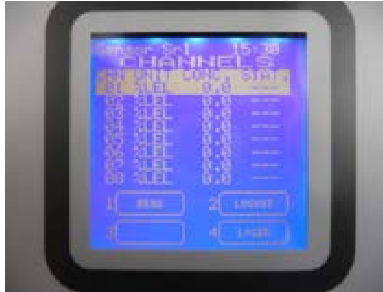
Figure 5.1.4 a) View Channels screen in "Operation" user level
