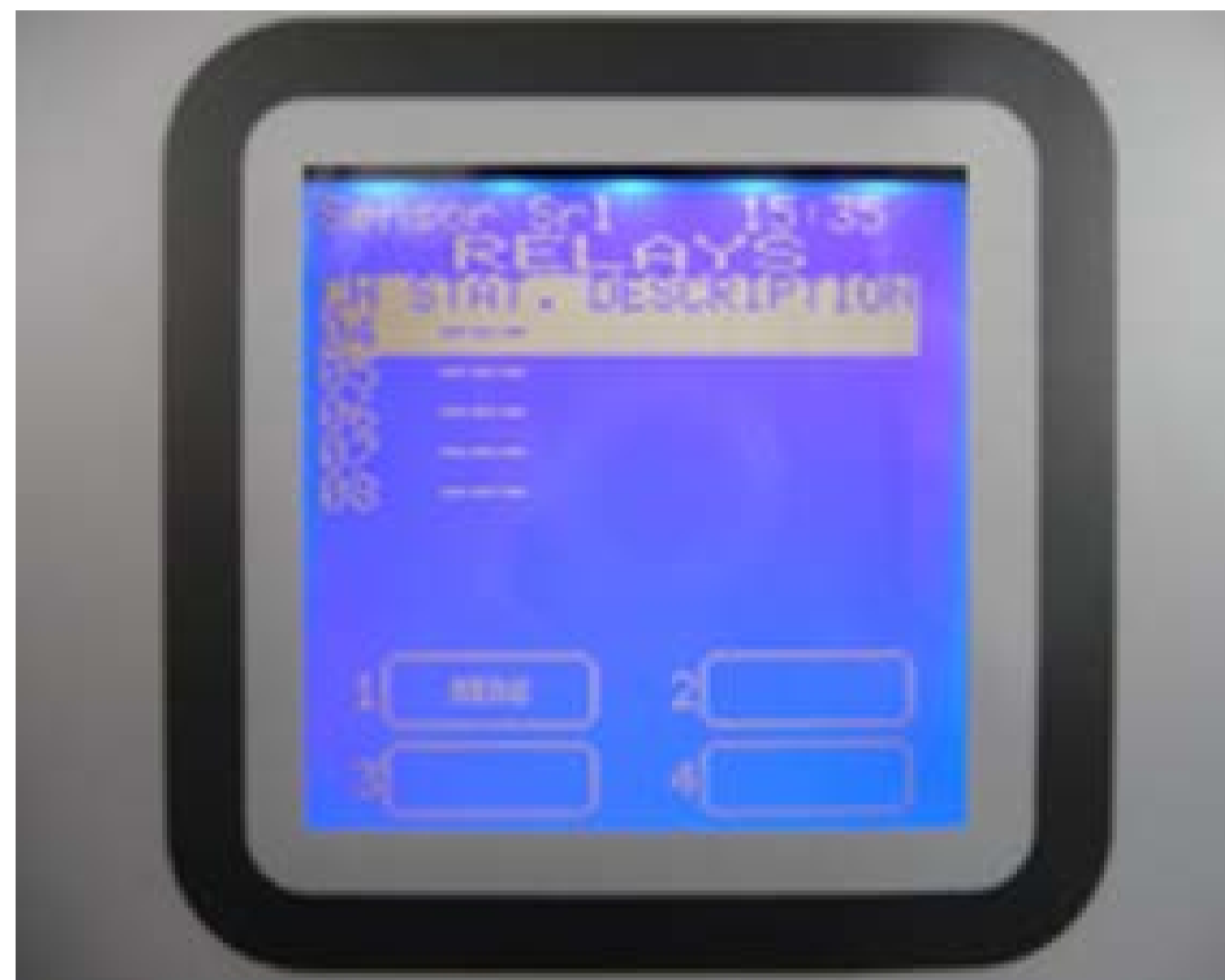
Figure 5.1.3 a) View relay screen in "Operation" user level
