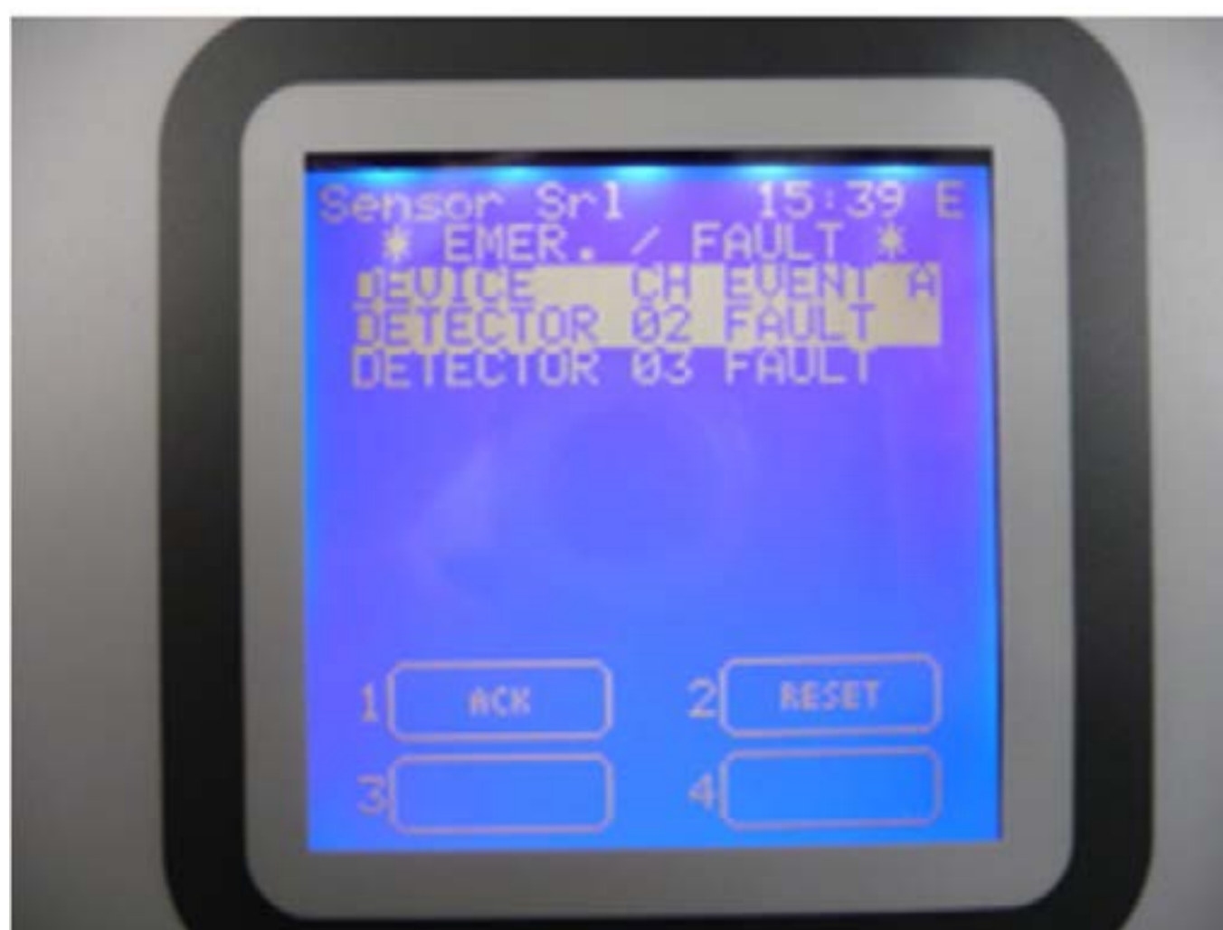
Figure 3.5 a) Typical FAULT state of the ACTIVE EVENTS screen.
