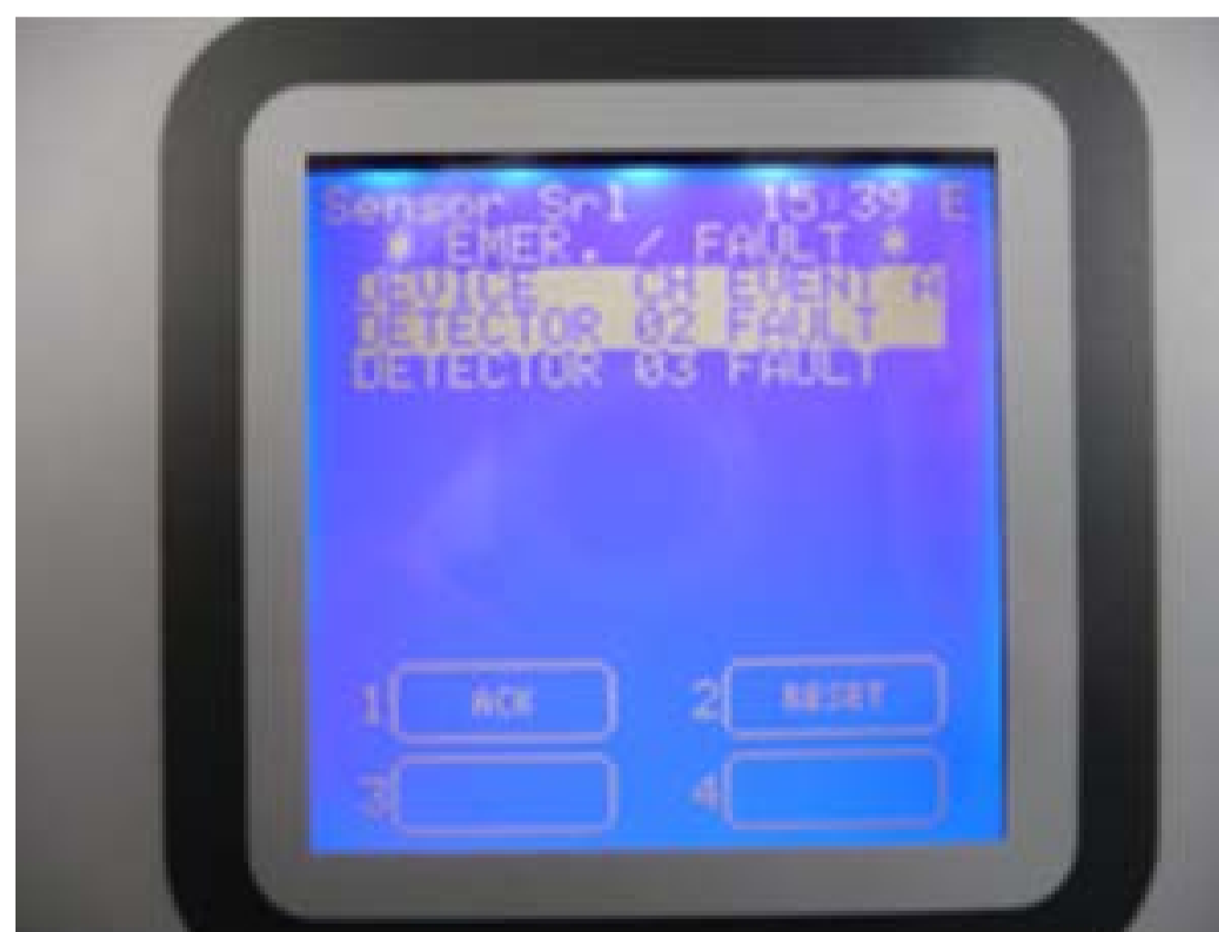
Figure 5.1.1 c) Active events screen with fault only
