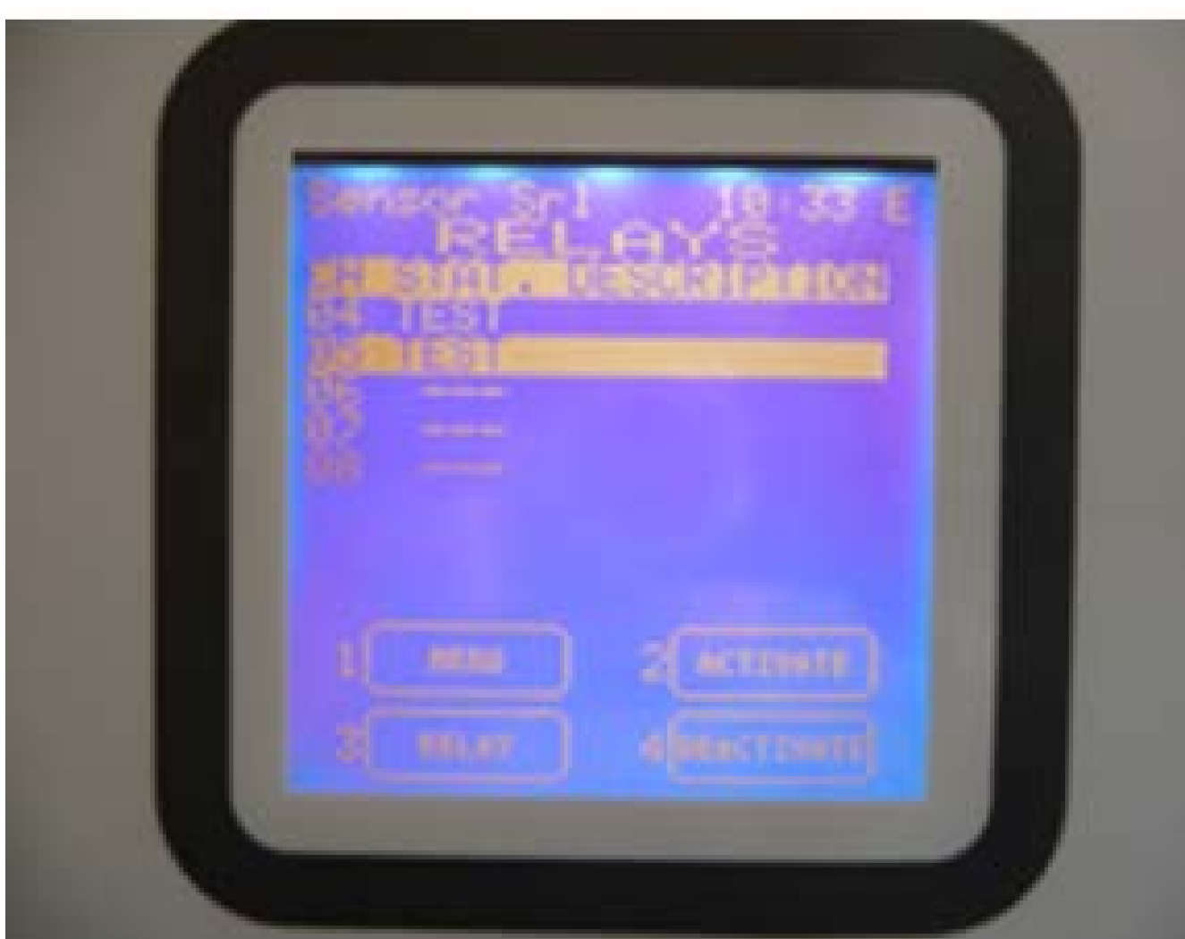
Figure 5.1.3 d) Screen with relays in “Test” status
