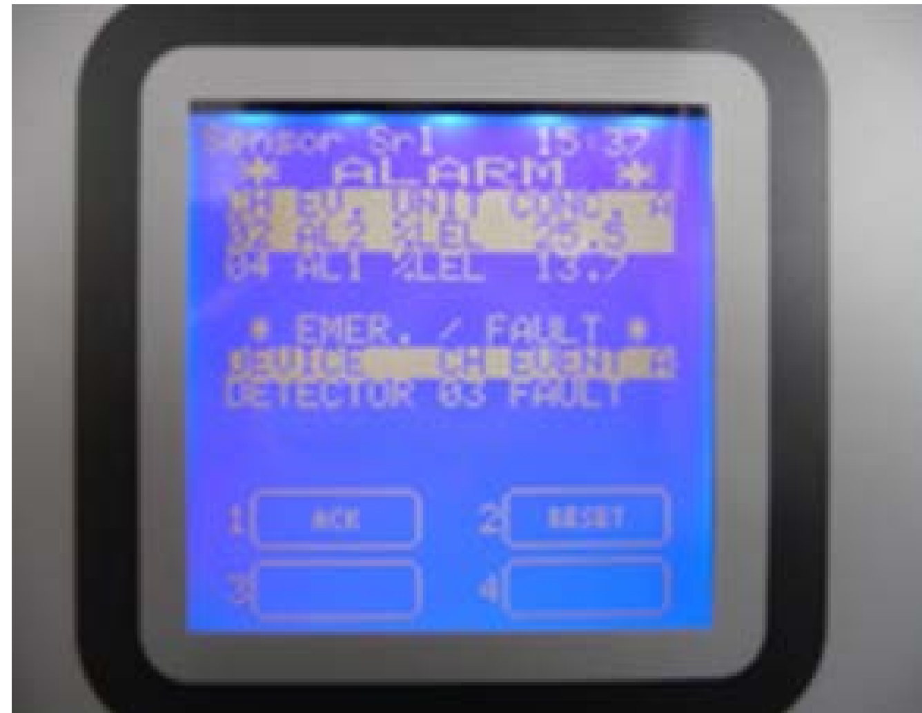
Figure 5.1.1 a) Active Events screen with Alarm and fault
